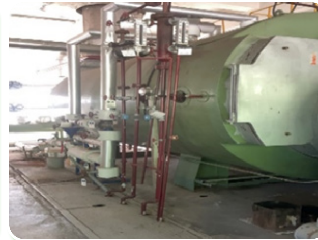
Equipment listed on the “Resource Exchange Platform”: Horizontal fire-tube boiler
