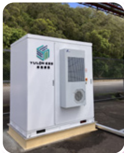
CUBE energy storage containers:
